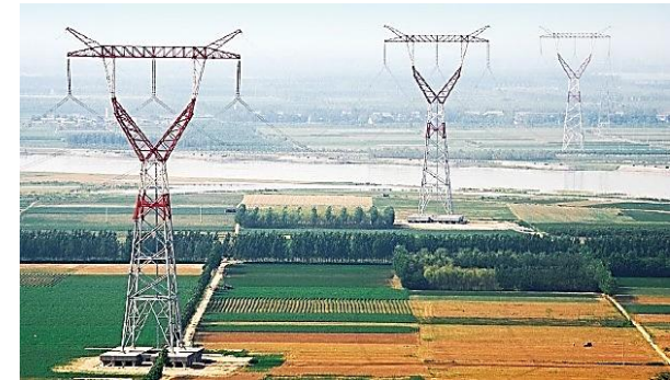
Jindongnan to Nanyang to Jingmen 1000kV UHV
